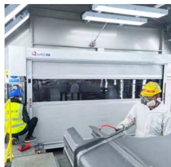
Painting Equipment Room
